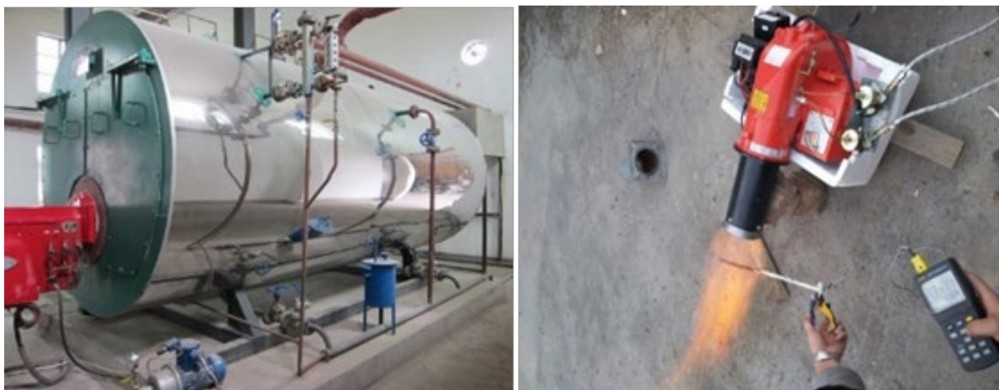
Figure 1-5 A 6 T/h Methanol Boiler for pharmacy plant and the burner in Xi'an
