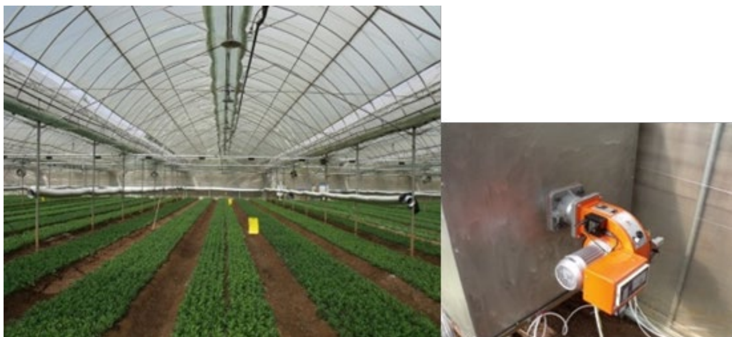
Figure 1-4 Methanol Boilers for a Flower Greenhouse and the burner
