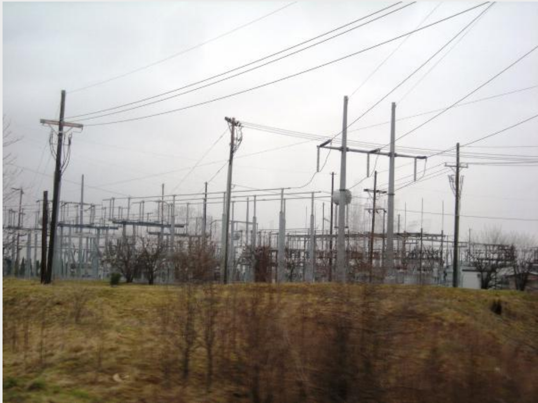
Increased Power Distributin in an Electric Car World. Hidden land use change.
